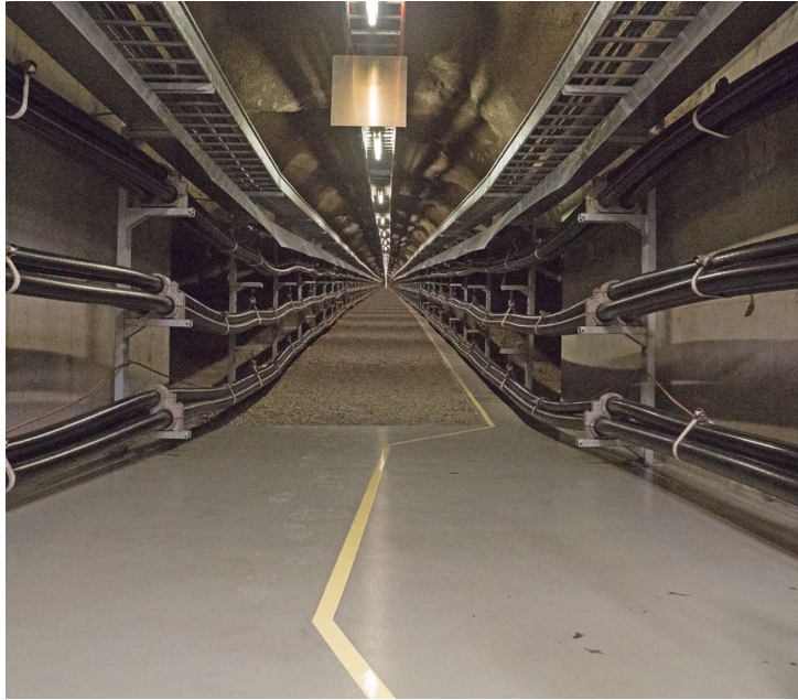
Photo 69: Fljotsdalur power station, cable tunnel
