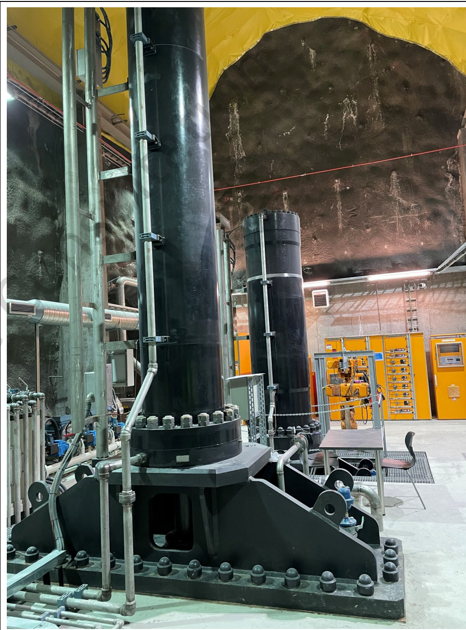
Photo 62: Bottom outlet gate at Kárahnjúkar Dam
