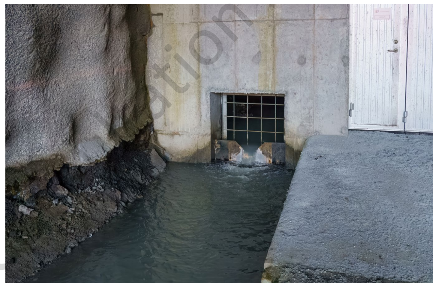
Photo 2: Drainage from headrace-tunnel leakage
